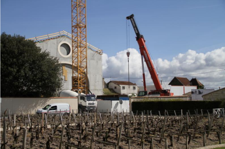
New cellar under construction at Mouton Rothschild to accommodate new gravitational presses, which are tried and tested to make finer wines.
